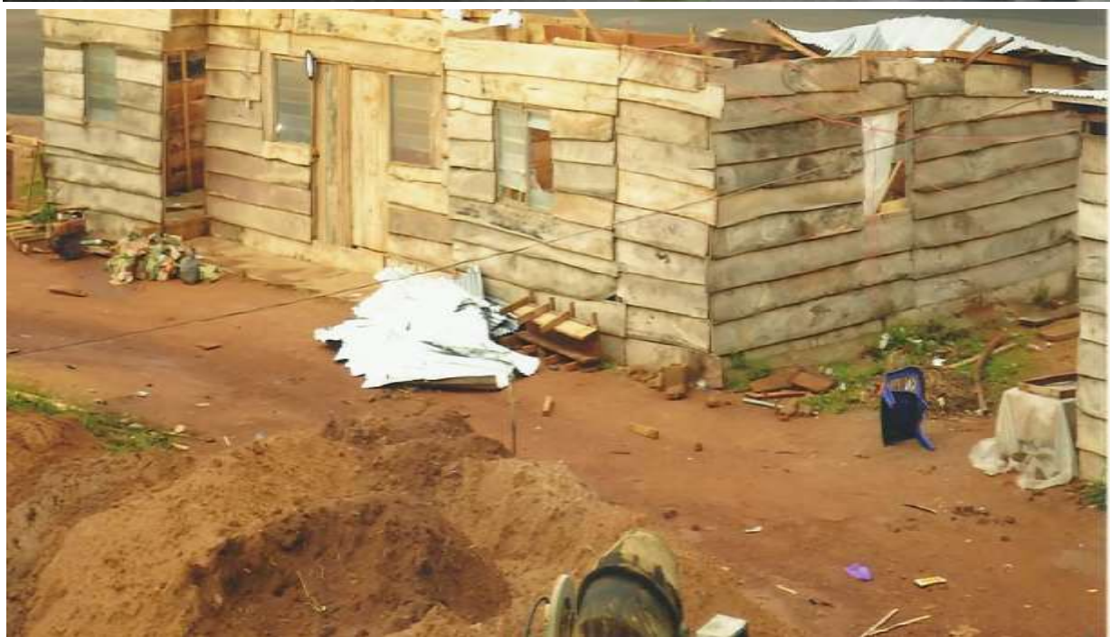
Pictures showing the removal of roofs on Buildings due to the Effects of wind.
